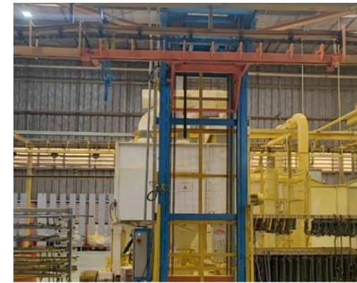
Elevator for Painting in Campo Grande
