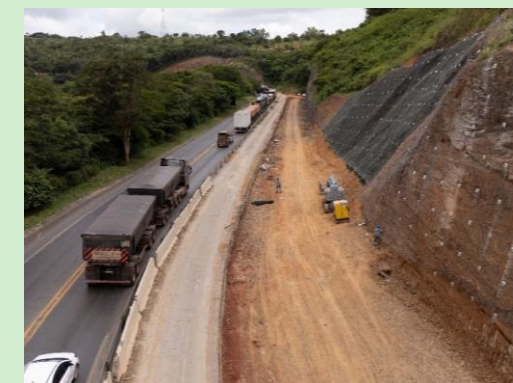
Eco135: road widening works between the municipalities of Montes Claros/MG and Bocaiúva/MG
