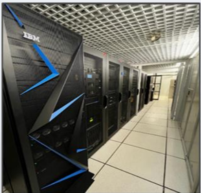
Server infrastructure update in 4Q23
