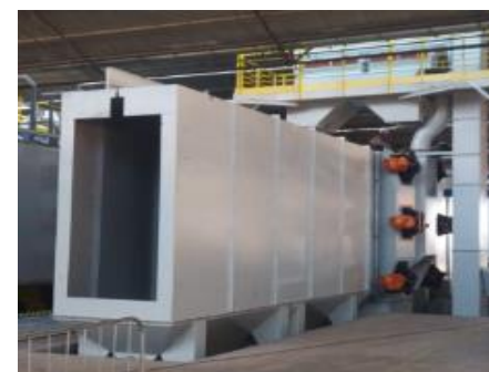
Powder Coating Line (Blasting Process)
